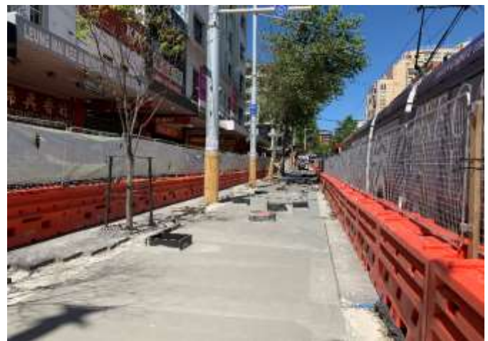
Concrete base ready for paving – George Street East side between Hay Street and Rawson Place
