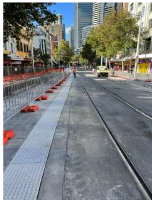
Tactile installation during Light Rail shutdown – George Street between Ultimo Rd and Rawson Pl (west side)
