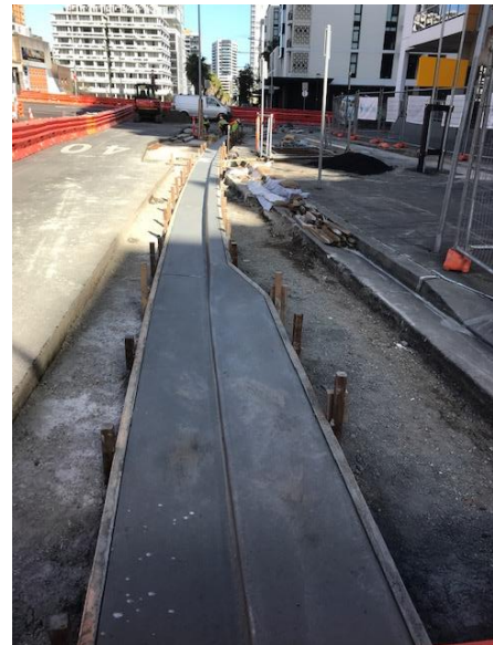
Photo above – Section of completed kerb and gutter section on the North West corner of the intersection
