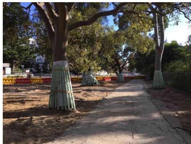
Photo above : Base for footpath on the Wollongong Rd end of the site.
