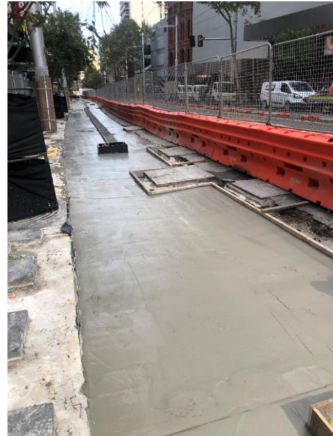
Concrete base – East side of George St between Bathurst St and Liverpool St complete (ready for paving).
