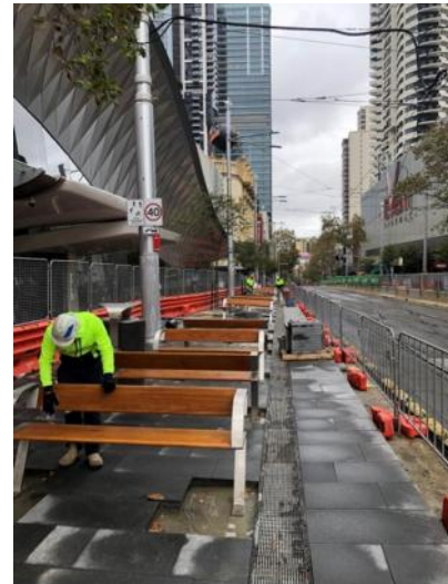
Paving and seat installation – East side of George St between Bathurst St and Liverpool St .
